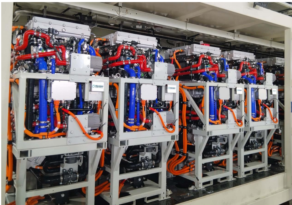
Horizon 2MW CHP “under the hood”
